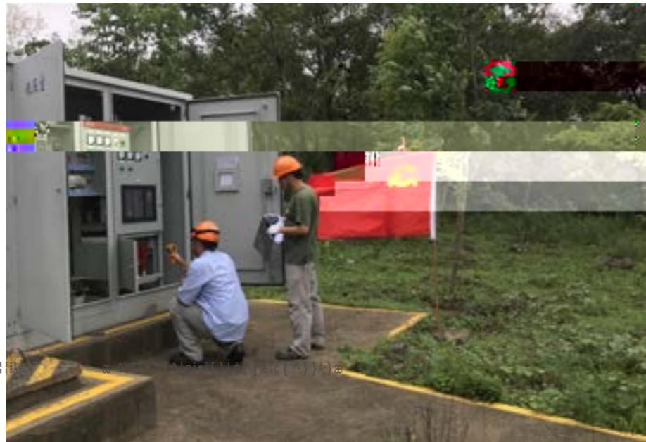
On the eve of the Super Typhoon Lekima's landing, the wind farms of Longyuan Jiangsu Company carried out special inspections to investigate and eliminate hidden troubles.
